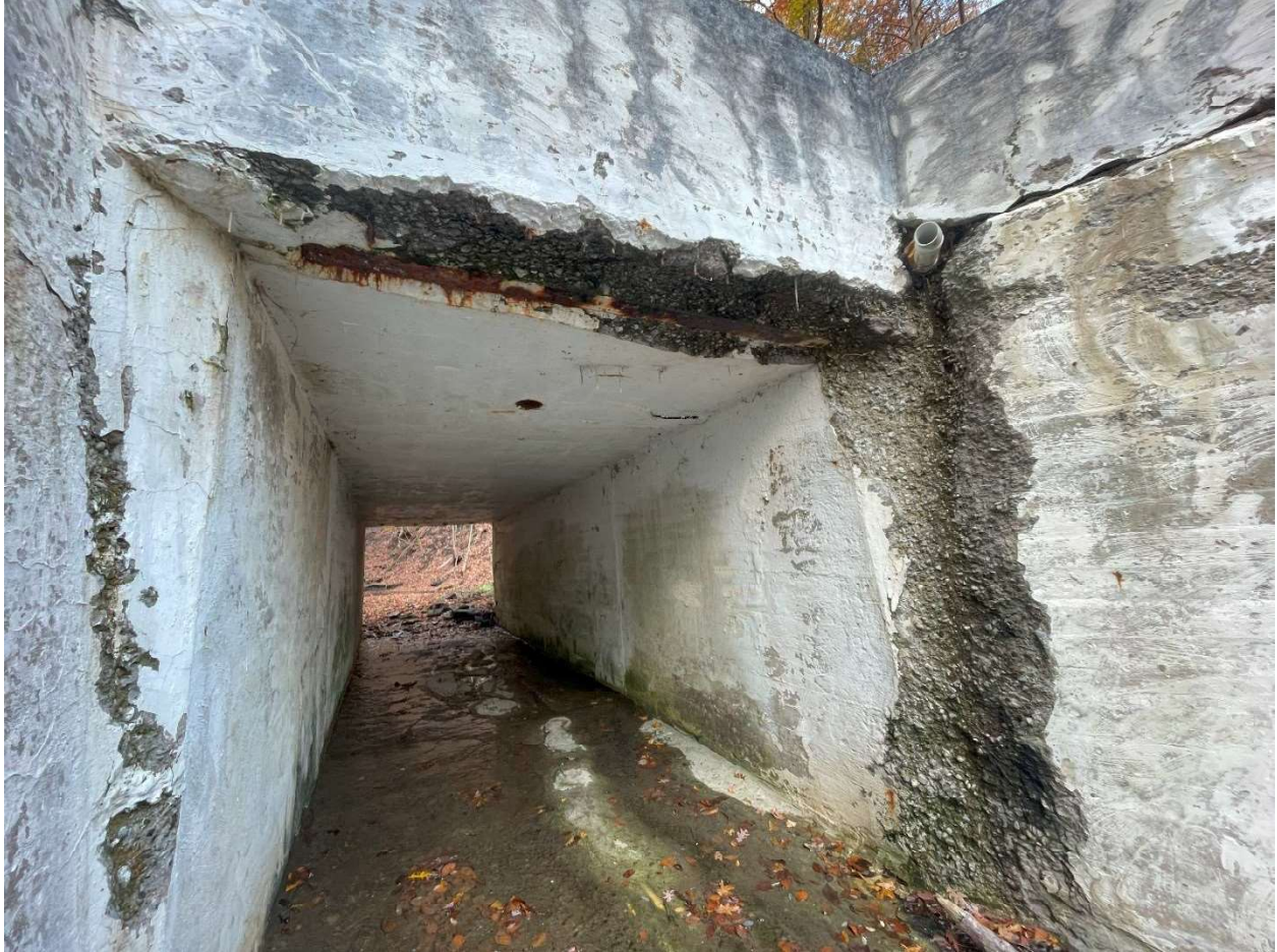
Figure 3. Maplewood Road culvert looking west. Spalling concrete with steel reinforcement exposed and corroding.
