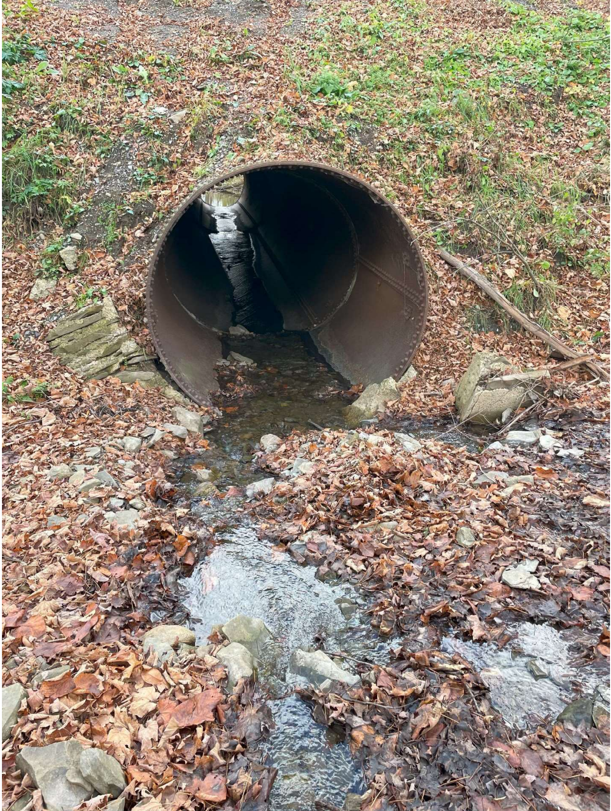
Figure 24. Iradell Road culvert looking north. Limited embedment throughout the culvert.
