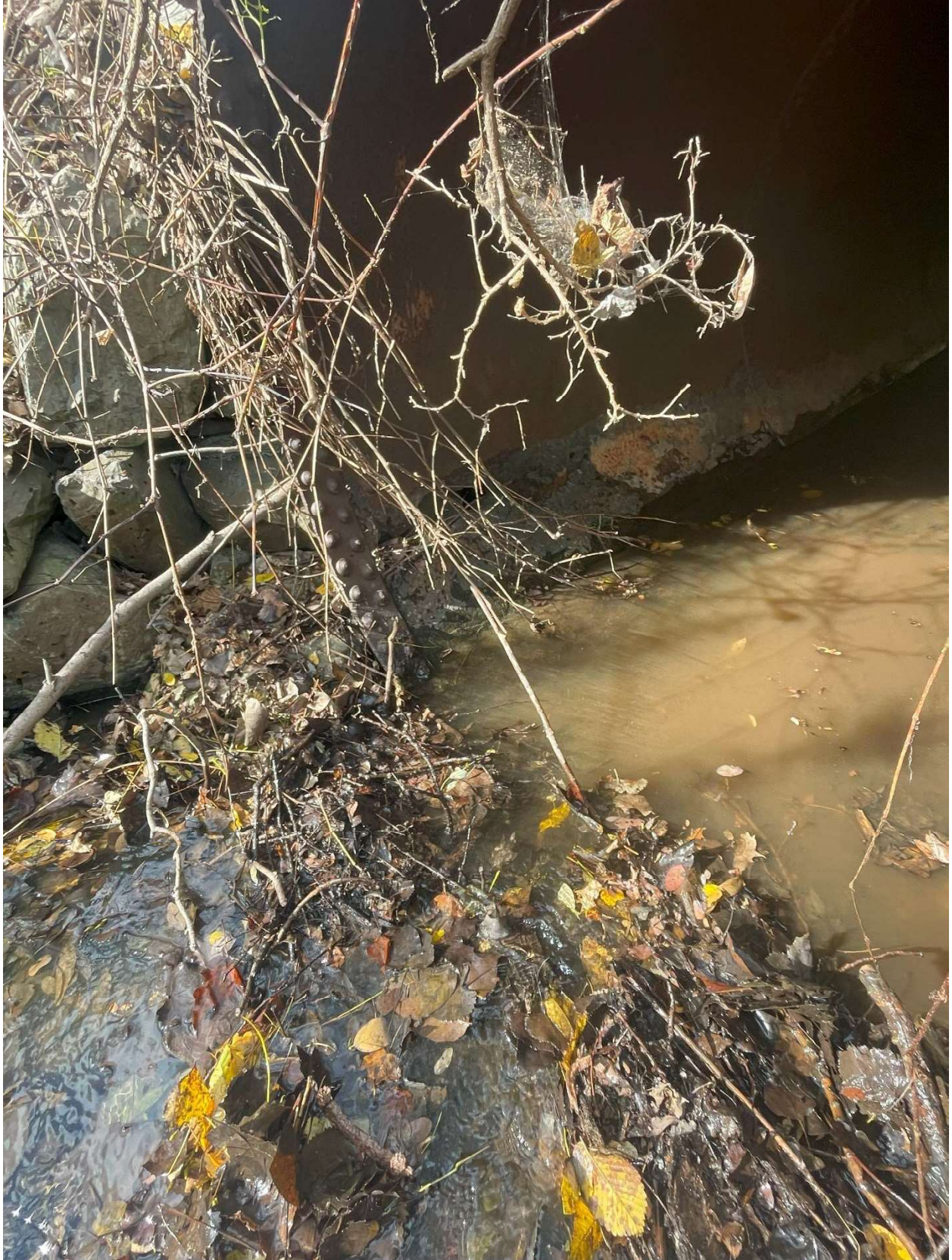
Figure 21. Corrosion on the inside of one of the Reynolds Road culverts.
