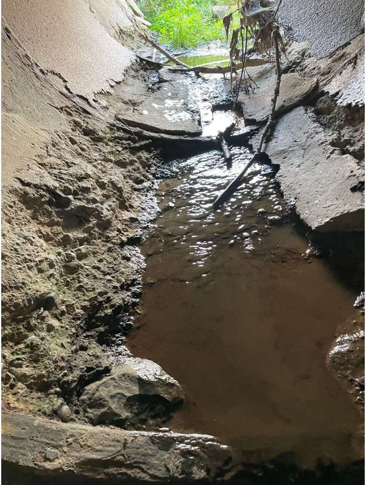
Figure 9. Garrett Road culvert looking west. The concrete on the bottom of the culvert is spalling.
