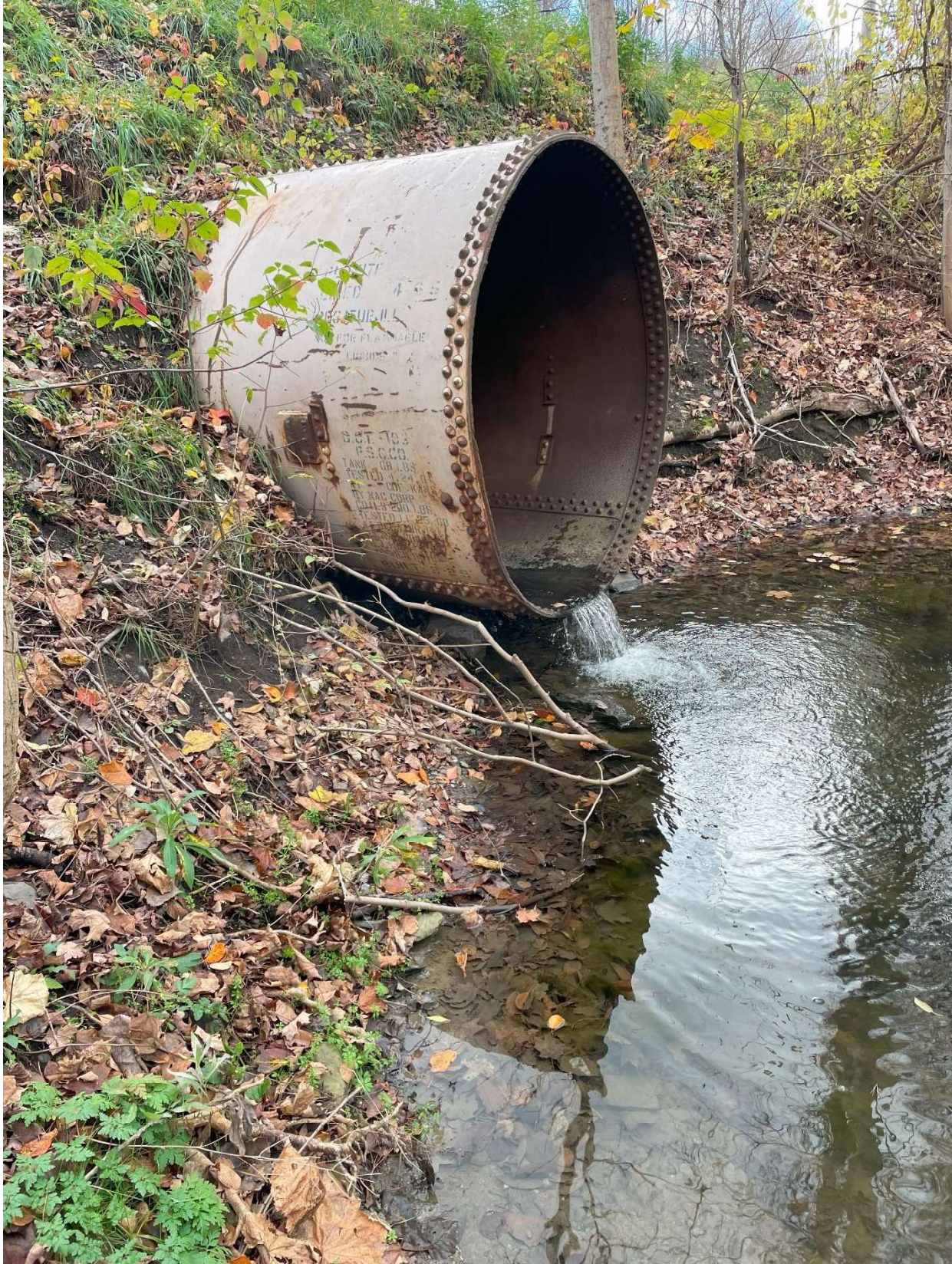
Figure 26. Iradell Road culvert looking southwest. Large vertical separation between the outlet invert and the streambed below.
