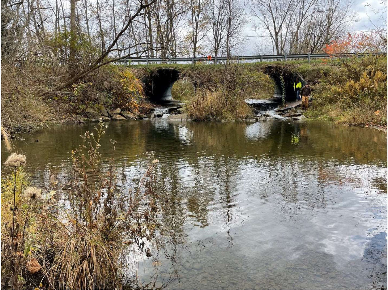
Figure 14. Curry Road culverts looking south. Large vertical separation between the outlet inverts and the streambed below.
