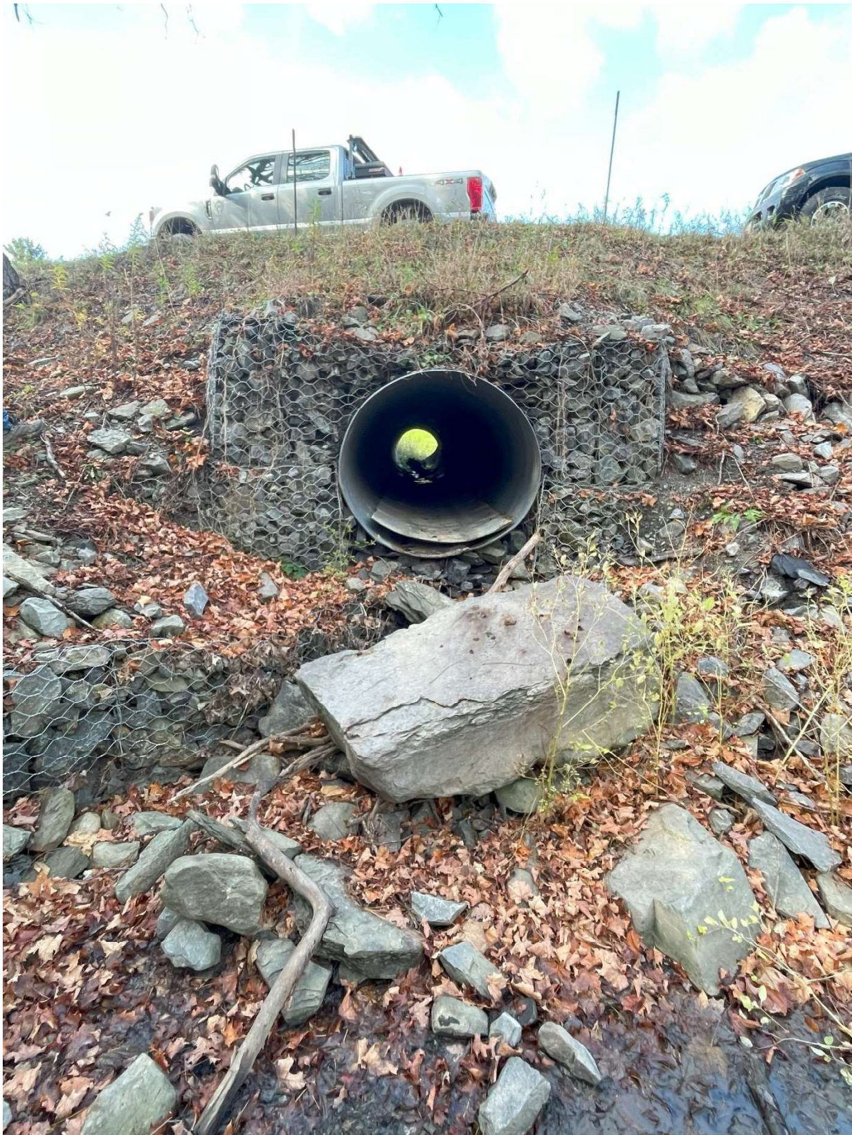
Figure 7. Garrett Road culvert looking west. Large vertical separation between the outlet invert and the streambed below.
