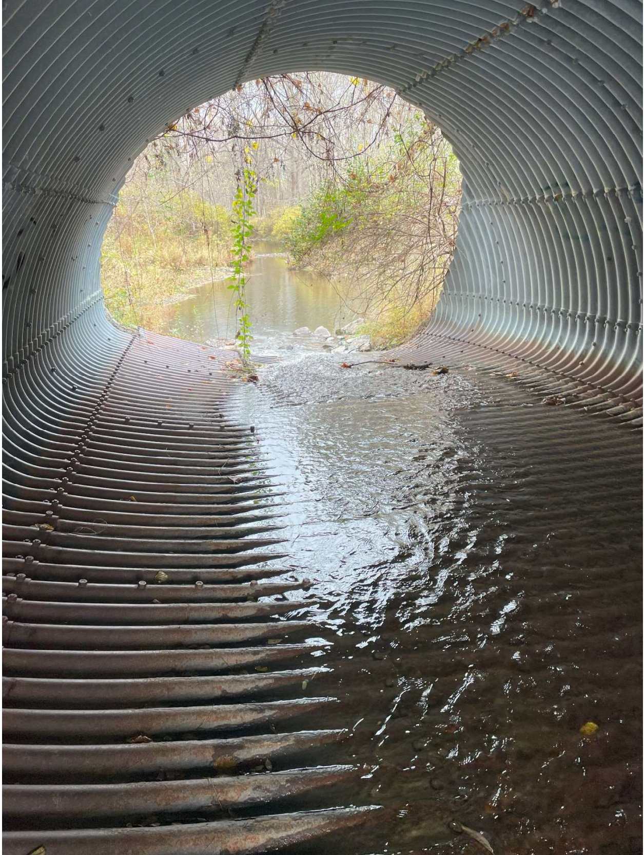
Figure 13. Curry Road west culvert looking north. No embedment throughout the culvert.
