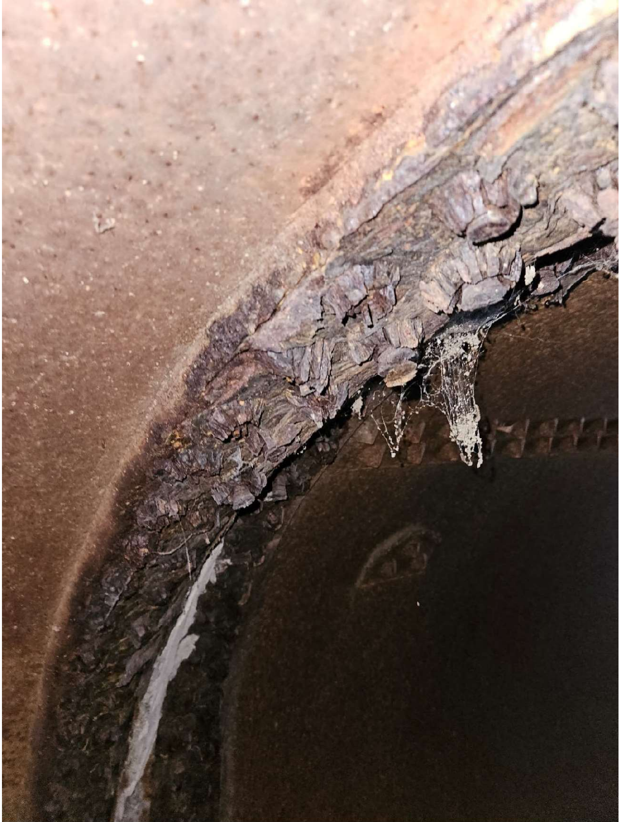
Figure 20. Corrosion on the inside of one of the Reynolds Road culverts.
