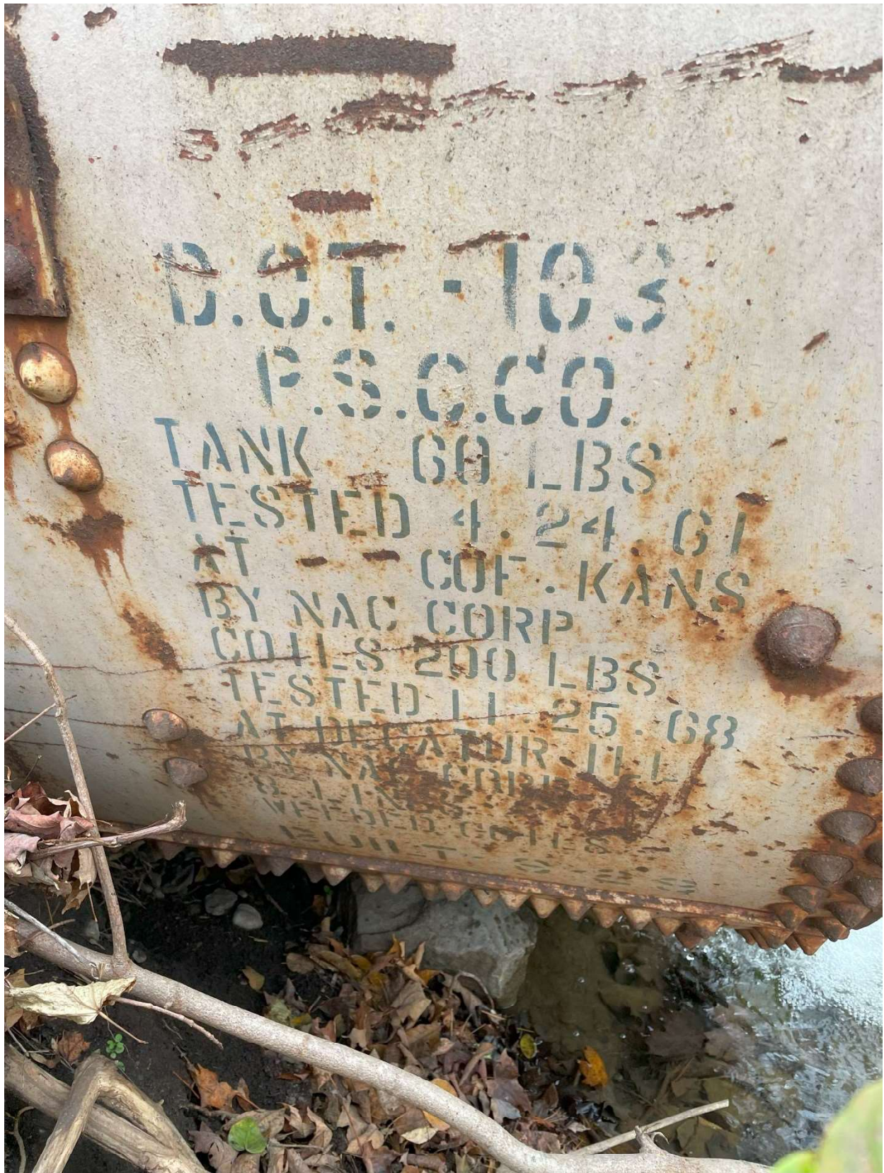
Figure 27. Iradell Road culvert looking at the outside of the culvert on the north end. The culvert appears to be made from an old freight car petroleum containment vessel.
