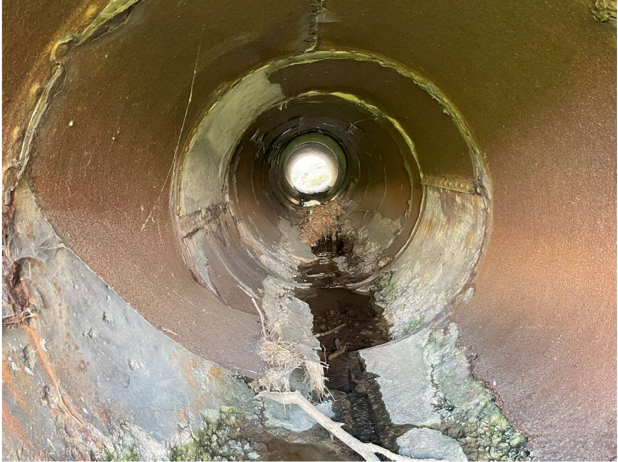
Figure 8. Garrett Road culvert looking east. The metal liner on the inside of the culvert is heavily corroded.
