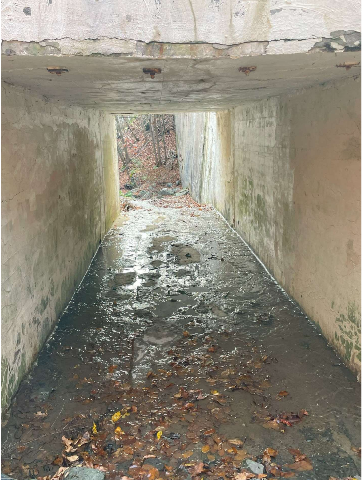
Figure 1. Maplewood Road culvert looking east. No embedment throughout the culvert.
