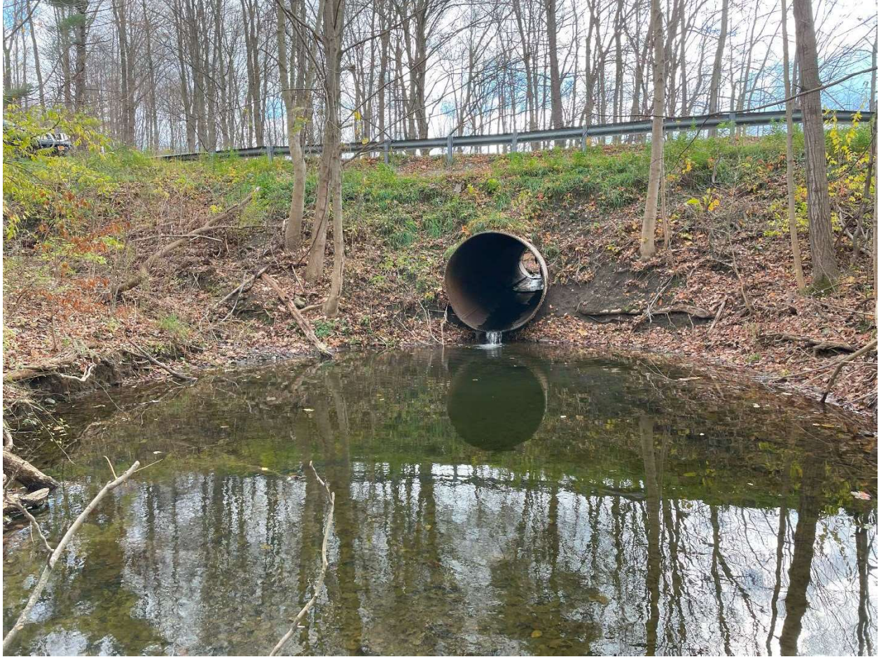
Figure 28. Iradell Road culvert looking south. There is a large pool forming at the outlet side of the culvert.
